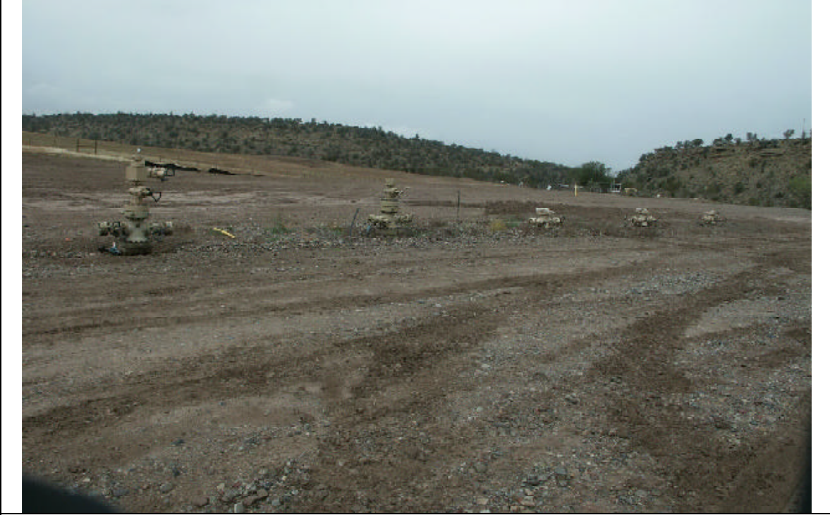
Figure 8. Five producing wells on the EnCana P3 pad. North is to the right, and the Magic 10-1 well is on the left.
